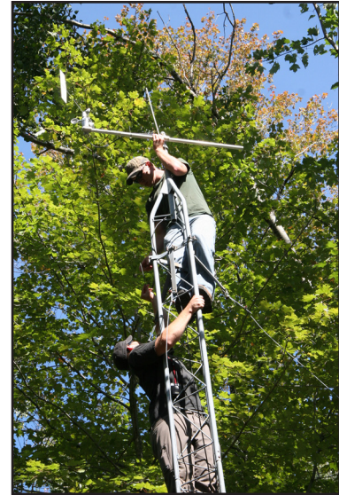
UWSP students are involved with every portion of the Schmeeckle monitoring station. Here, two students install the wind vane at the top of the tower.
