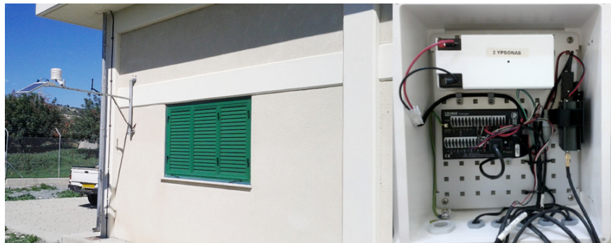
CR200 connected to Apogee SP-110, Pyranometer and Campbell 109
