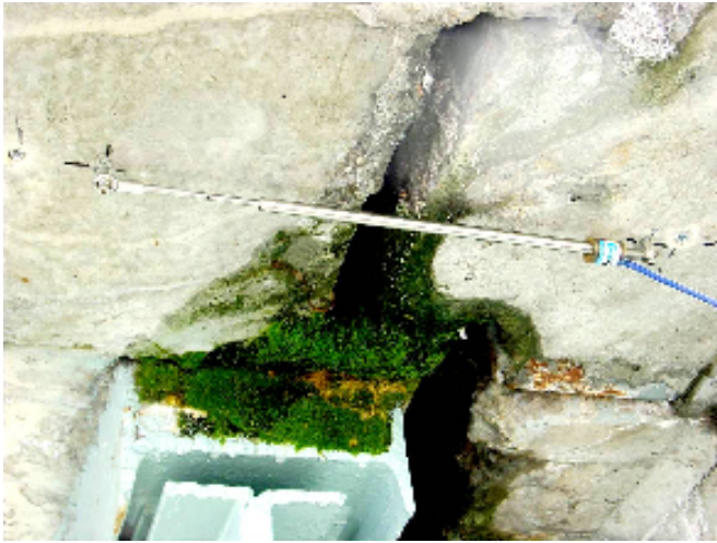
Fig. 1: Vibrating Wire Extension Gage on an Expansion Joint
