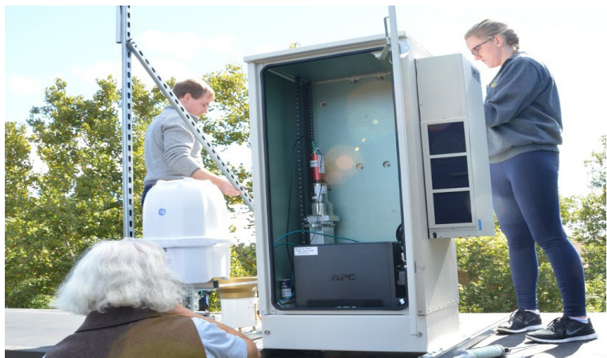
Configuration on the rooftop. The enclosure was mounted to the rooftop, with the data logger and backup power supply inside, and the GE Gamma Radiation Monitor, TE Precipitation Monitor, and Vaisala Weather station to the left of the enclosure.
